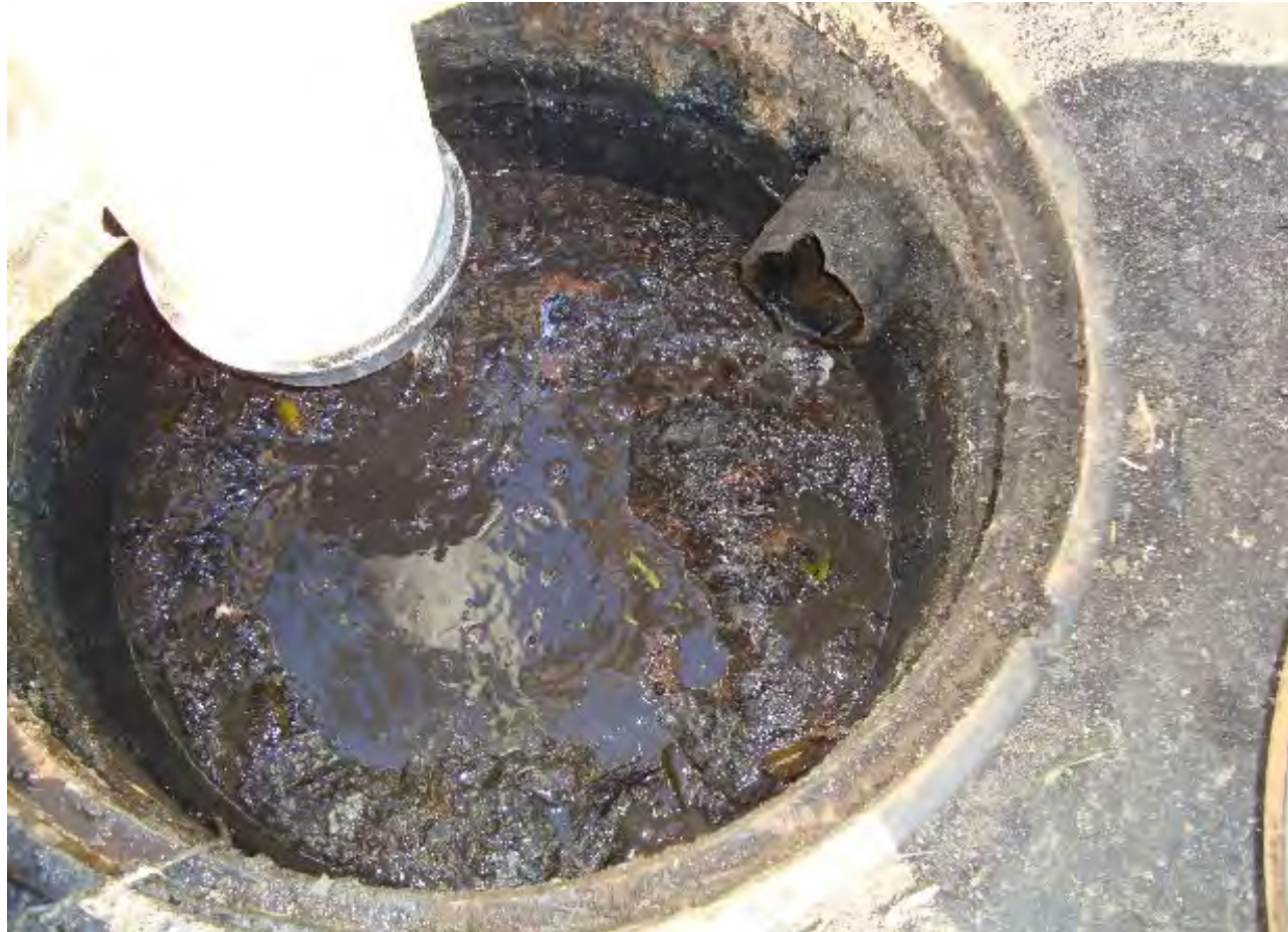
Sanitary Discharge, Private Storm Drain
